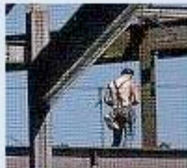
Personnel Safety Netting
